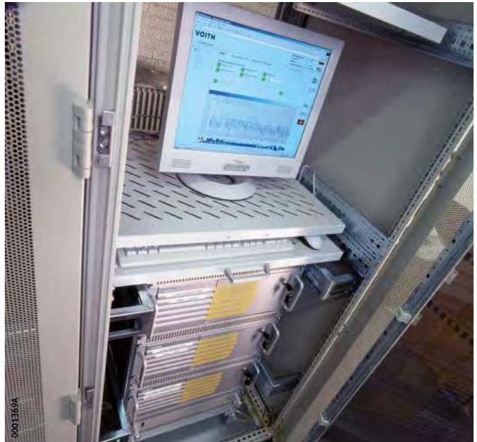
Figure 10 Condition-based rolling bearing monitoring using FAG VibroCheck
